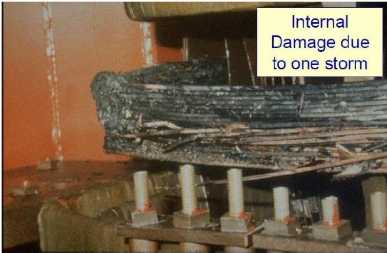
Damaged Core on Salem Nuclear Power Plant Transformer
